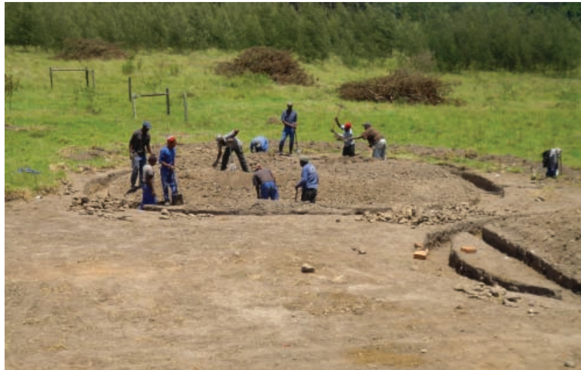
LOCAL WORKERS DIG THE FOUNDATIONS BY HAND AS THEY BEGIN CONSTRUCTION ON THE FIRST THREE COTTAGES
